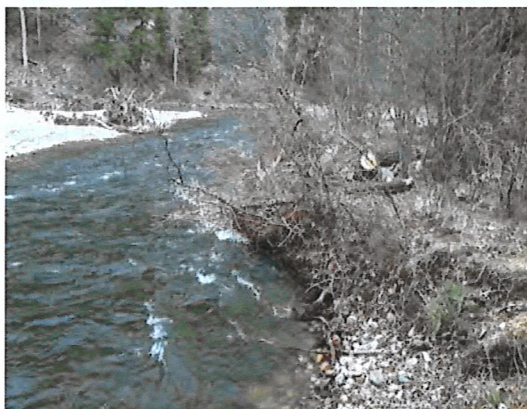
Projects to stabilize eroding streambanks require a 310 permit.
