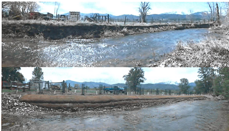
Pre and post construction of double vegetated soil lift on Rye Creek
