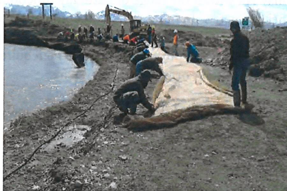
Geotextile bank treatments can be labor-intensive. Backfilled brush layer in place, ready for first soil lift.
