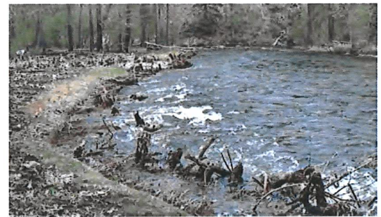
A completed soil lift with large woody debris toe emulates the natural range of bank roughness and stability.
