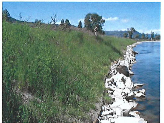
This site used rock to stabilize the toe, however, brush or woody debris would have been equally effective and preferred.
