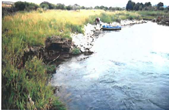
Receding bank upstream of a rip-rap job will eventually lead to failure.
