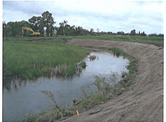
Stream banks are sloped to a 1.5:1 or 2:1 angle and covered with biodegradable geotextile fabric. Toe protection is frequently brush or willow layers. Same location as above photo.
