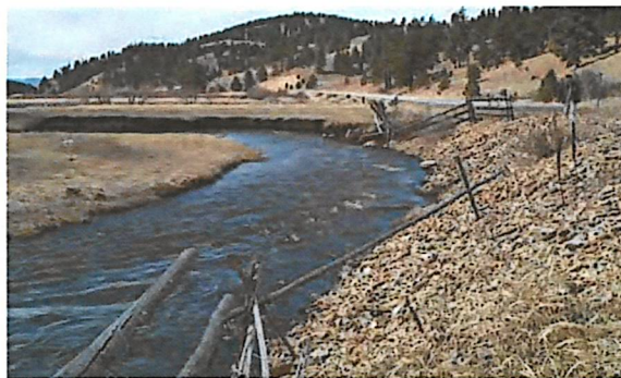
A well designed rip-rap job has 2:1 slopes and does not encroach on the river. This bank may have been stabilized using geotextile and vegetative methods with equal success. Note that Erosion has moved downstream below this rip-rapped bank.
