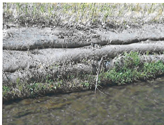
In low erosion/scour locations, toe protection may be “soft” techniques such as coir logs or biodegradable fabric lifts.
