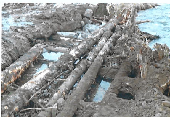
A robust toe protection technique relies on large woody debris to provide a high degree of scour protection.
