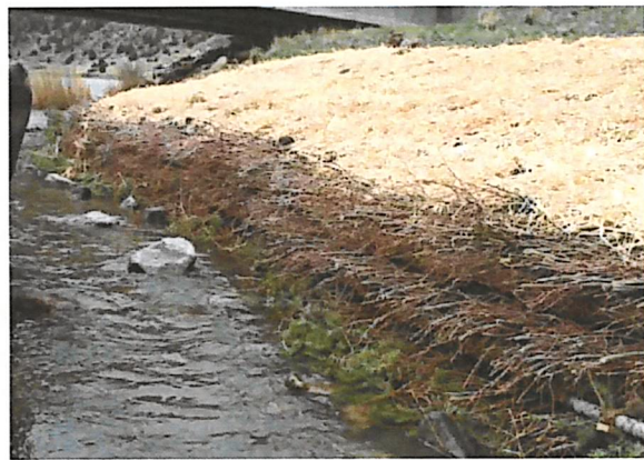
A conifer fascine toe with three soil lifts provide contextually appropriate treatment to stabilize this bank on the Madison River.
