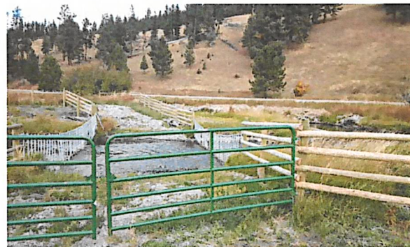
A hardened crossing provides a discrete area for livestock to access the stream and additional pastures. The swinging flood gate placed across the water with drop PVC pipes allows for high flows and debris to pass.
