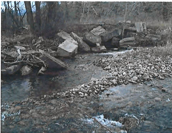
Concrete is generally not acceptable for large angular rock rip-rap. Contact Montana DEQ for guidance regarding use of concrete as rip-rap.
