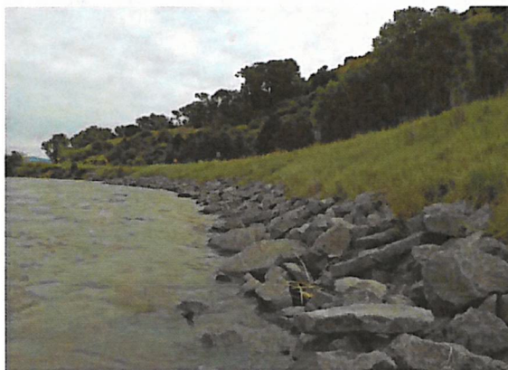
The upper bank stabilized with natural geotextile fabric has been successfully revegetated for aesthetic value. Incorporating willows within the rip-rap can further enhance natural processes.
