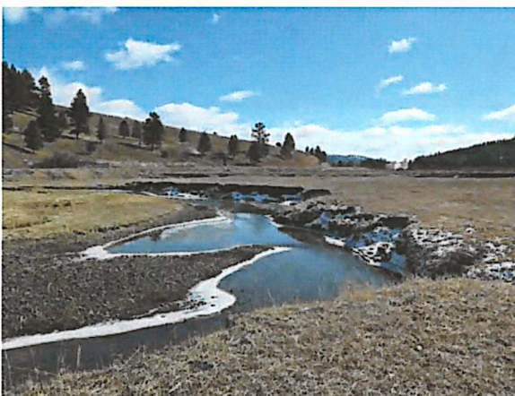
Poor Condition: accelerated bank erosion, high width to depth ratio, migrating channel location, large and irregular sediment deposits
