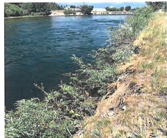
This bioengineered bank is deforming as the river undercuts the encapsulated soil lifts. Deformable banks are frequently incorporated into restoration strategies, but may be undesirable for structural protection.
