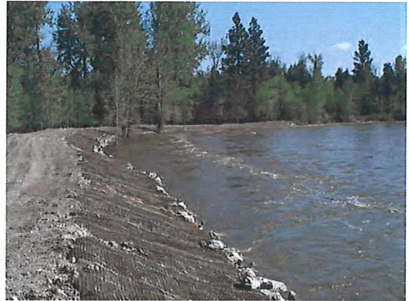
This dike was stabilized to protect downstream development from flooding, although the landowner with the dike did not particularly want to constrain the river.
