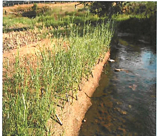
Creating an appropriate moisture regime is key to establishment of wetland and riparian species. Willow cuttings should be placed deep enough to intercept the water table.
