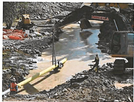
Flowing water through a construction site can result in severe water quality impacts. Potential sediment release must be addressed during the permitting process.
