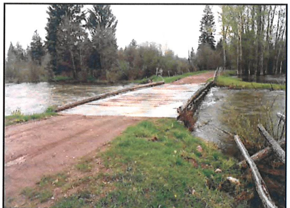
This bridge stringer is also a good indicator of bankfull. Projects should avoid this situation, which traps debris.
