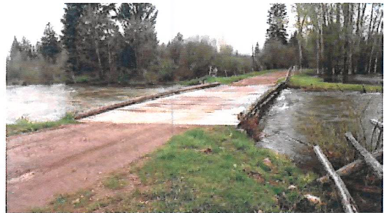
Stream crossings on shallow channels with broad floodplains must rise to meet the bridge, or the bridge will end up being too low, like this one.
