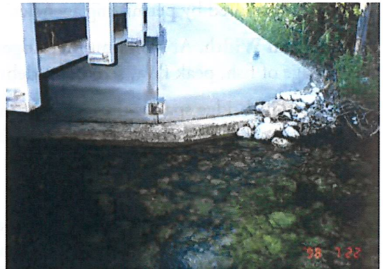
Concrete can make good abutments, provided the footing is placed below scour depth. This footing should be 2 feet lower.
