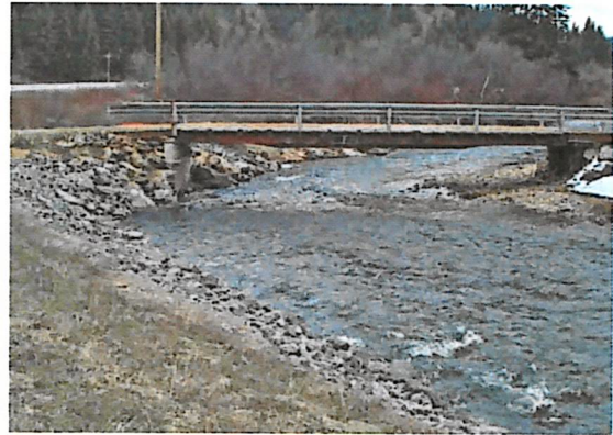
This bridge is set slightly above bankfull, but does not have wingwalls. Location on a meander is not ideal, although upstream rip-rap limits lateral movement. Note, point bar is still growing under bridge.
