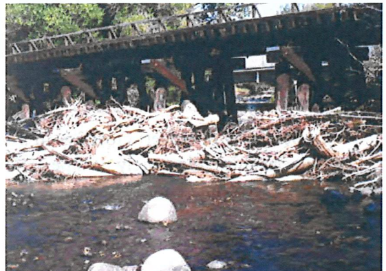
Debris jams are often associated with center piers on bridge crossings. A clear span is preferable to piers.
