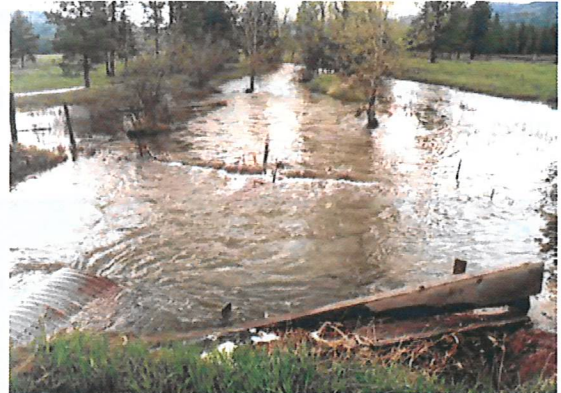
This undersized culvert caused large amounts of gravel to deposit in the channel upstream. Woody debris must be cleaned frequently from the inlet.
