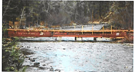
Railcar bridges are popular and fairly solid, but often are not installed properly. This one is set low relative to bankfull, but it is a temporary installation.
