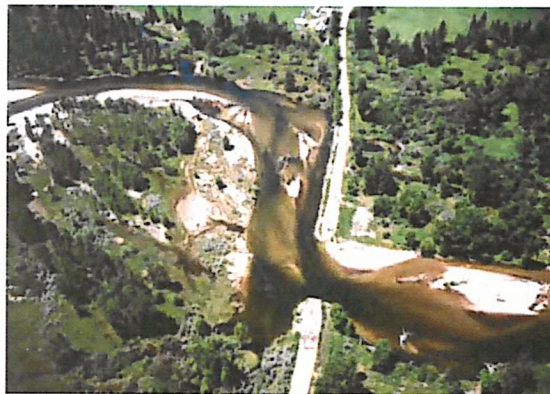
Choosing a location with a stable cross section is critical to project success. This failed bridge had inadequate span and was located on an actively migrating river reach. Over time, the river migrated to the west (top of photo) and the bridge location no longer matched the river alignment.
