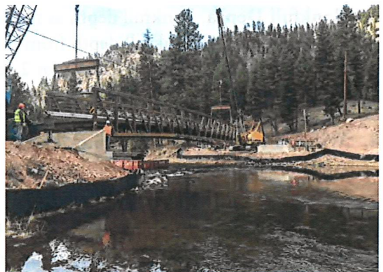
Concrete abutments are generally preferred, and must be protected from scour at the toe. Note the silt fence in place during construction to minimize turbidity.
