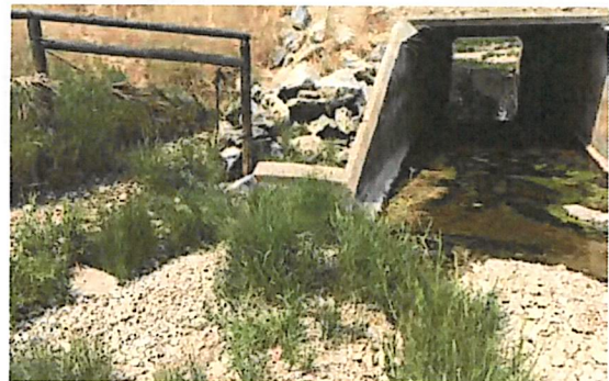
A well-designed box pipe enables fish passage by retaining a natural channel bottom substrate.
