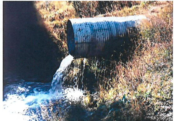
The shotgun (or perched outlet) culvert impedes fish passage, and can result from placing the culvert too high, or installing the culvert in a channel that has a tendency to downcut without grade control downstream of the outlet.
