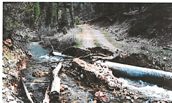
Undersizing pipes to save money is a poor strategy.
