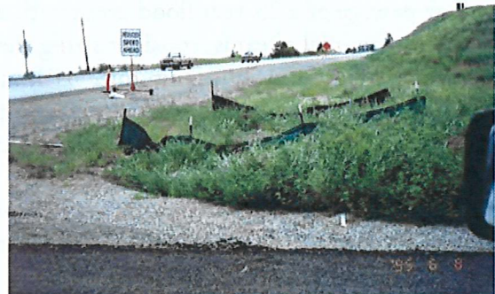
Silt fence helps prevent sediment delivery on newly constructed roads, but does not substitute for proper drainage features.
