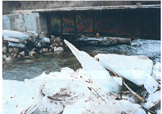
This bridge stringer was set below bankfull, and had problems with ice jams and flow capacity.
