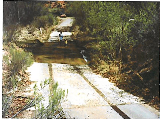
Fords may be a viable alternative for intermittent channels or channels that are shallow and wide and resist other solutions.
