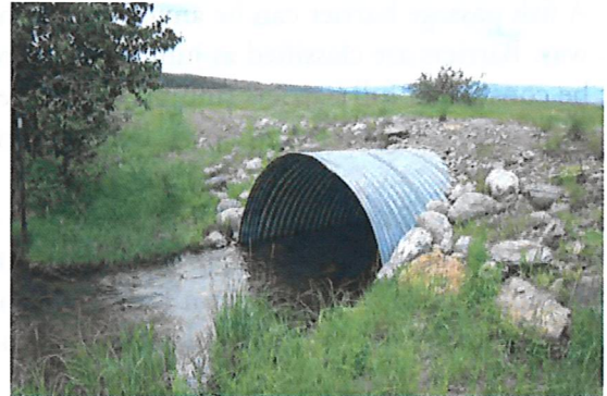
A well designed culvert allows for passage of flood events, and ideally, retains channel substrate material in the culvert to promote fish passage.
