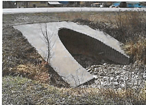
This arch pipe is sized to carry the predicted 25-year flow, but causes backwater at the 100-year flow.
