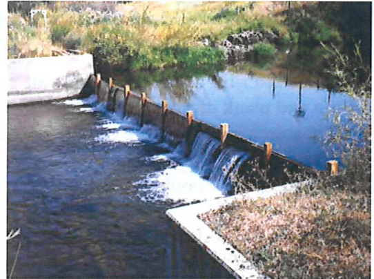
Concrete may be preferred to wood for longevity. This structure is not fish friendly because of the height of the drop and the flat slab downstream.
