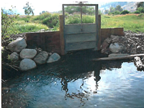
Careful design helps reduce impacts to the stream and cuts maintenance costs on irrigation diversions
