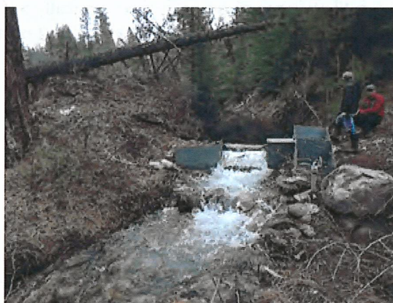
Fish screens can be installed in a stream, side channel, or ditch. Individual site constraints will dictate options that can be considered.
