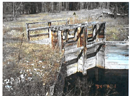
This is a well-constructed gate with wingwalls and positive control at high flows.
