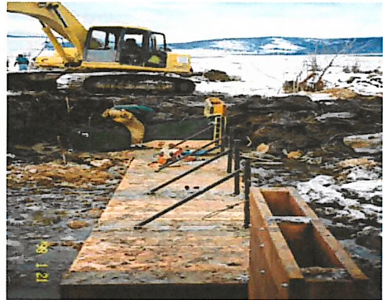
The flat floor and high drop of a pin and plank structure limits fish passage.
