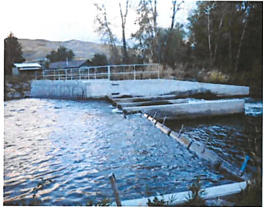
Inflatable bladder gates are generally used in specialized applications where precise control of water is important.
