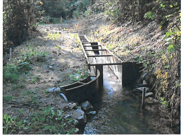
The screen entrance is in the background; foreground shows screened water on the right and bypass channel (fish return) on the left.
