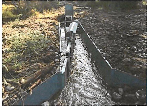
Vertical flat plate screens rely on paddle wheels to power the cleaning brushes. Bypass water returns young fish to the river channel.
