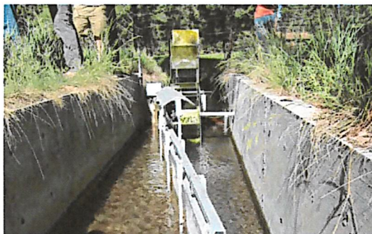
Fish screens are effective for preventing fish loss in irrigation ditches. A by-pass channel is normally needed to redirect fry to the main channel. A flat screen relies on brushes to clear debris.
