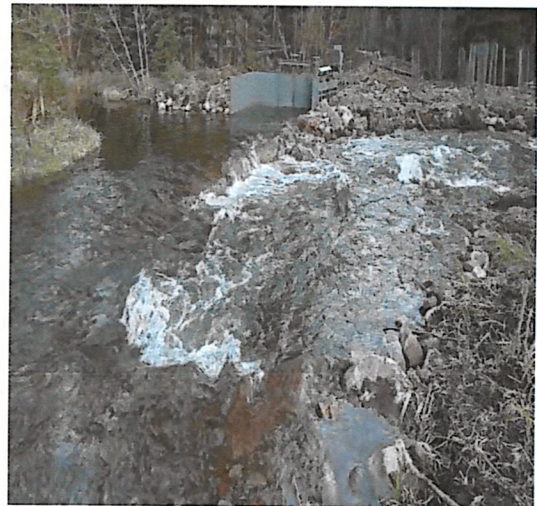
The diversion in the photo above was replaced with a engineered riffle structure, which allows fish passage and maintains natural stream processes.
