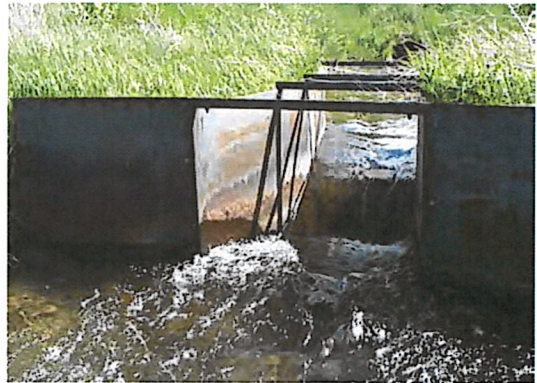
Parshall flumes cause minimal backwater, and work well in low-gradient applications.
